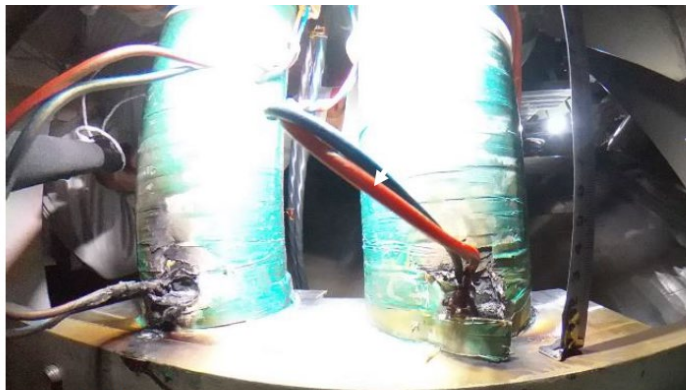
9 March 2021 – Double Fault to ground on EF coil terminals
