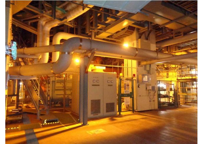
Piping developed to just underneath of the tokamak hall.
