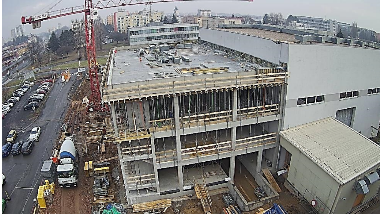
Three-floor new hall for power supplies, diagnostics and gyrotrons
