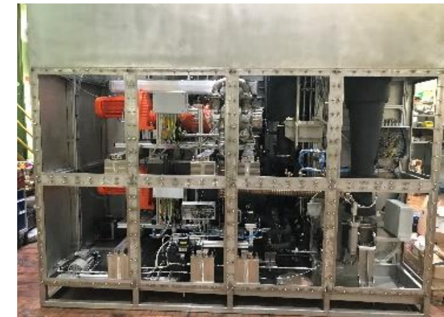
Arrangement of 2 ring pumps and 1 booster diffusion pump
